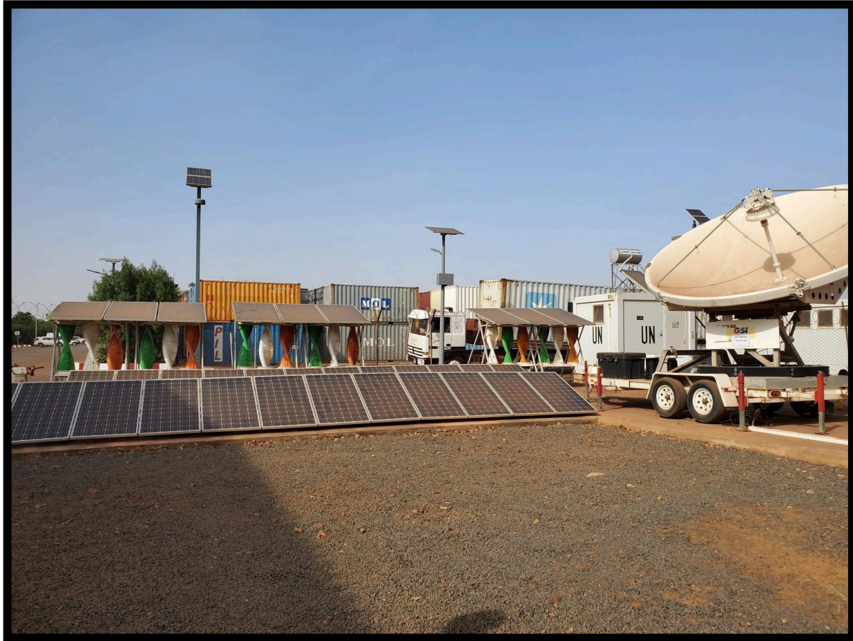
FIGURE 7: SATELLITE AND SOLAR PANEL INSTALLED IN UN FIELD MISSION
